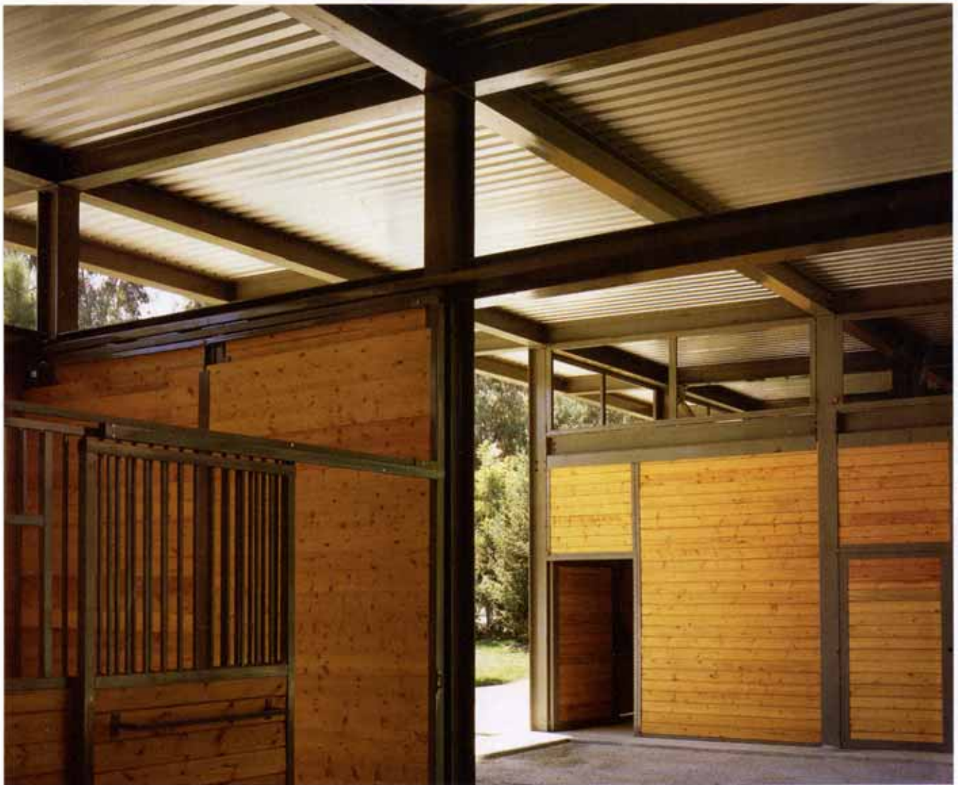
A 12-foot grid defines the structural system. The storage room (through door at right in photo) has a glazed clerestory, while the rest of the barn is open at the roof to ventilate the interior.
