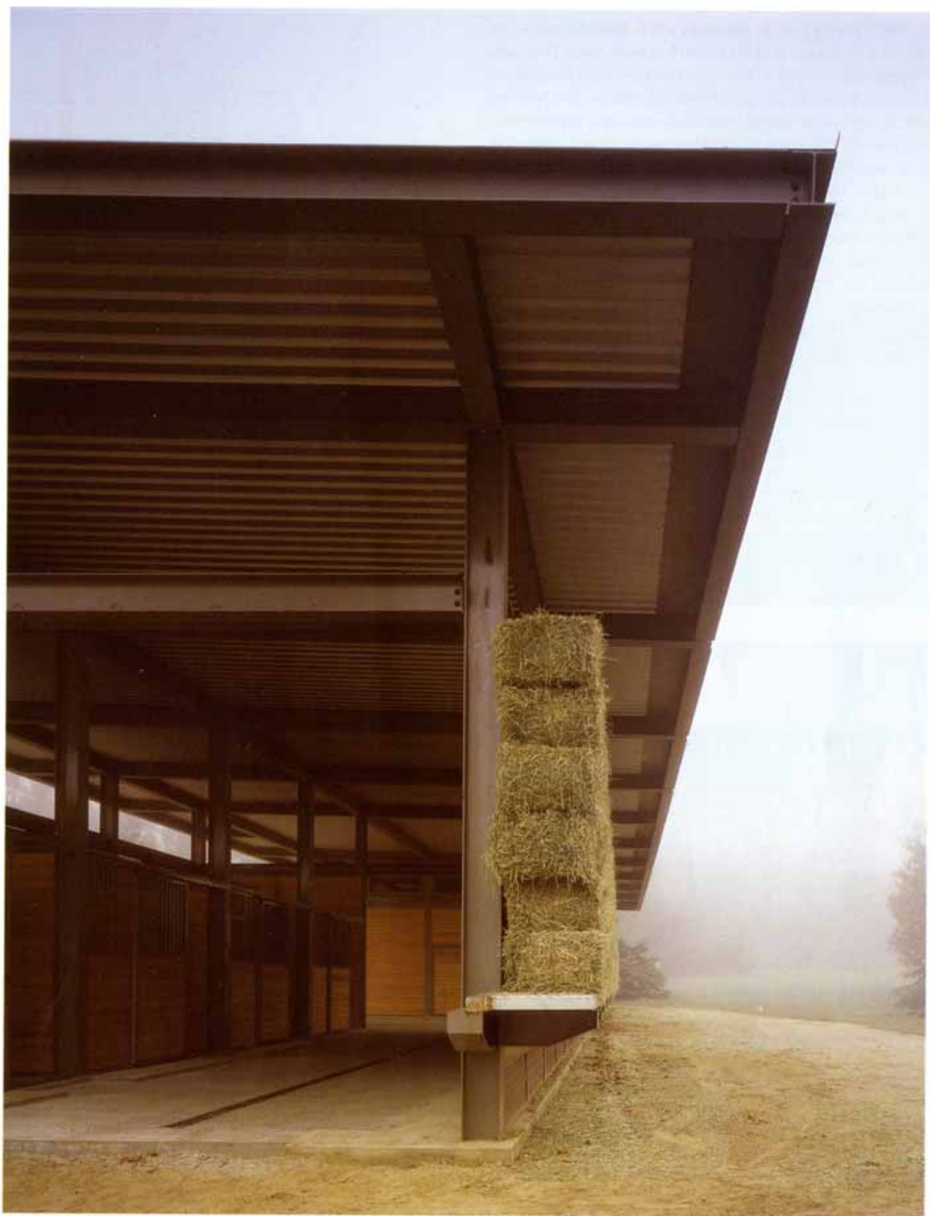
The barn holds four stalls and an enclosed room for farm equipment, feed, and tack. Hay bales are stored on a galvanized-steel grate supported by a painted-steel outrigger fastened to structural columns.
